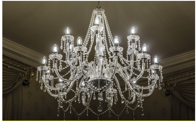
Integral LED filament lamps are installed in over 30 chandeliers at Wollaton Hall, Nottingham.
